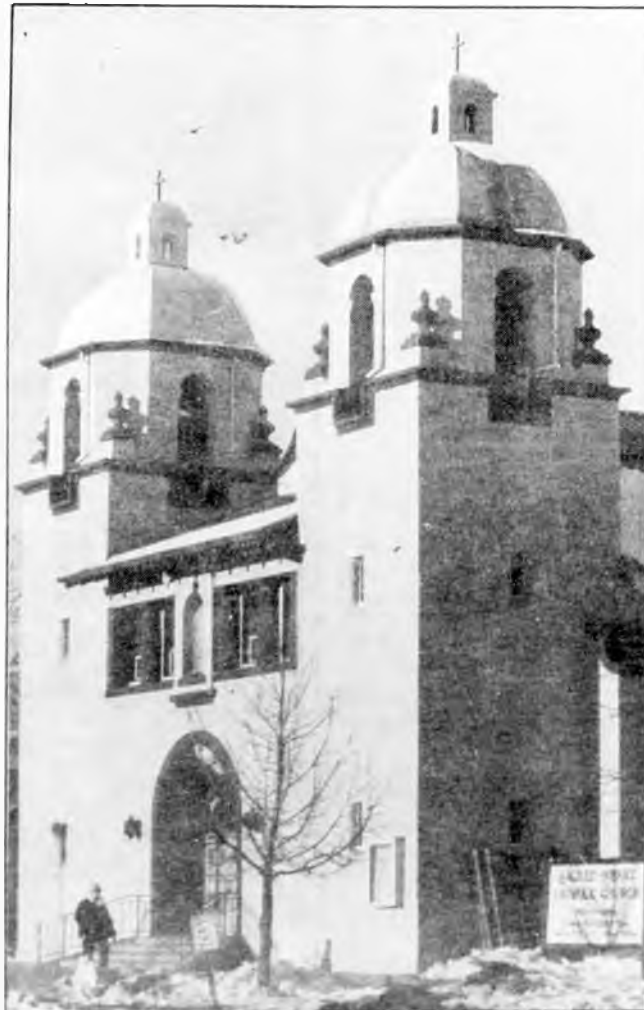
Sacred Heart Church at 21st and W. Colorado is nearing completion of its exterior restoration.
